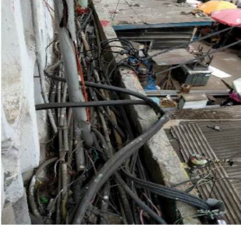
Figure 17. Detail View of Kerehida LV Network
