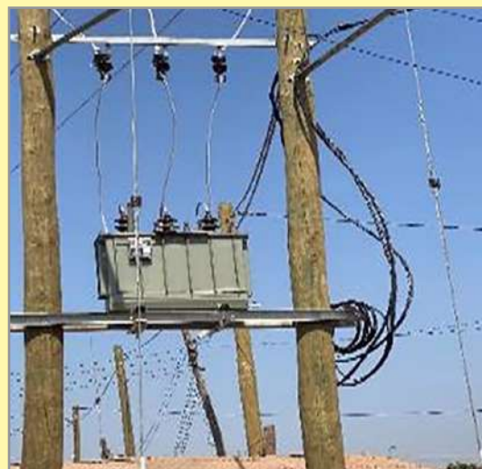
MV Network and Transformer Installation
