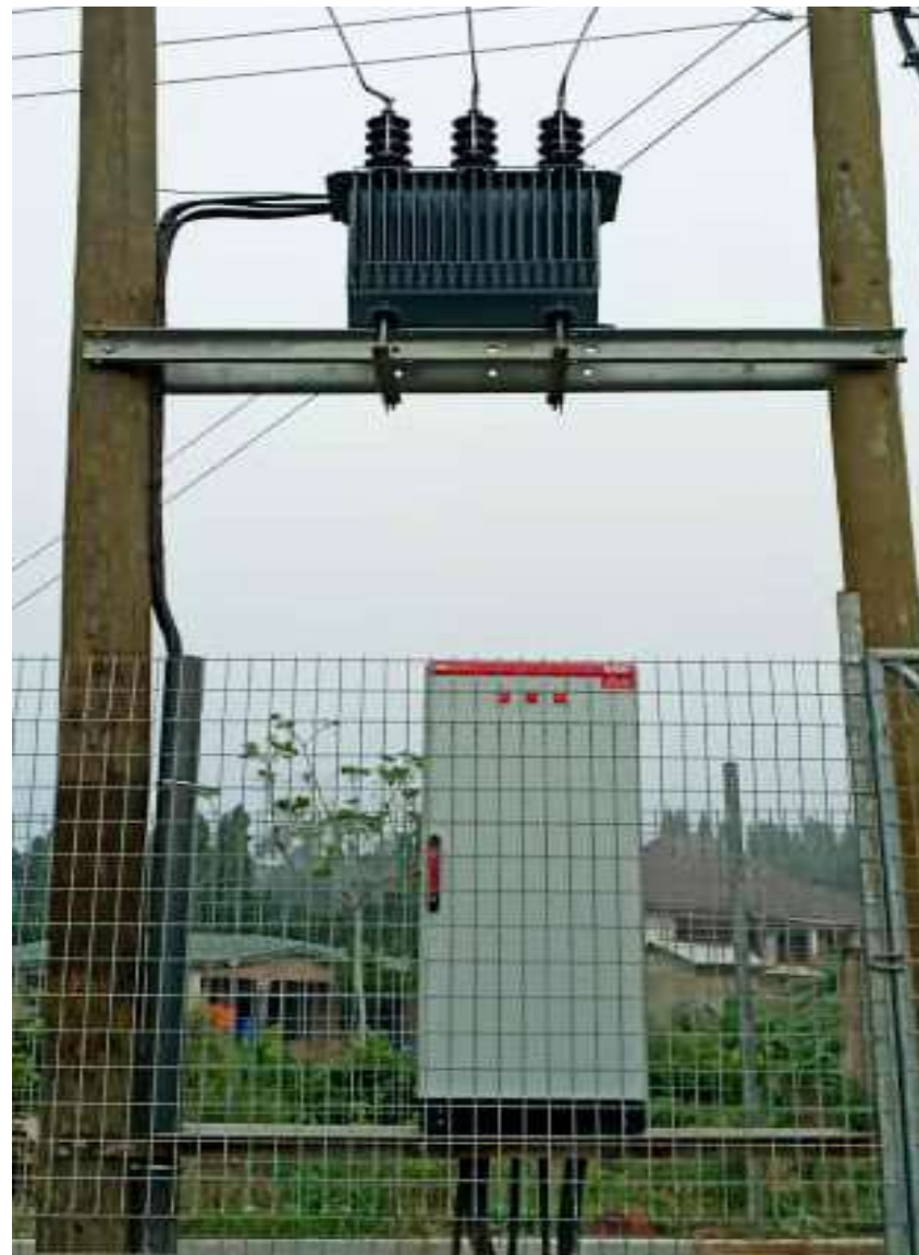
One of several Transformers and Ring Main Units installed in Akuapem Mampong District
