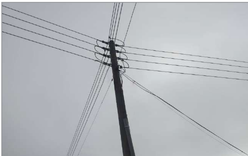
An upgraded low voltage line in Dansoman District
