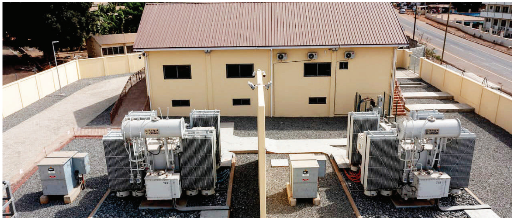
A view of the Ellen Moran Primary Substation - Kanda
