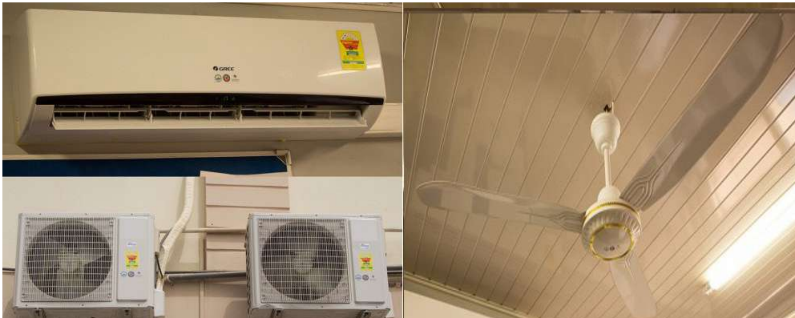
Energy efficient air conditioners and fans installed at the Korle-Bu Teaching Hospital.
